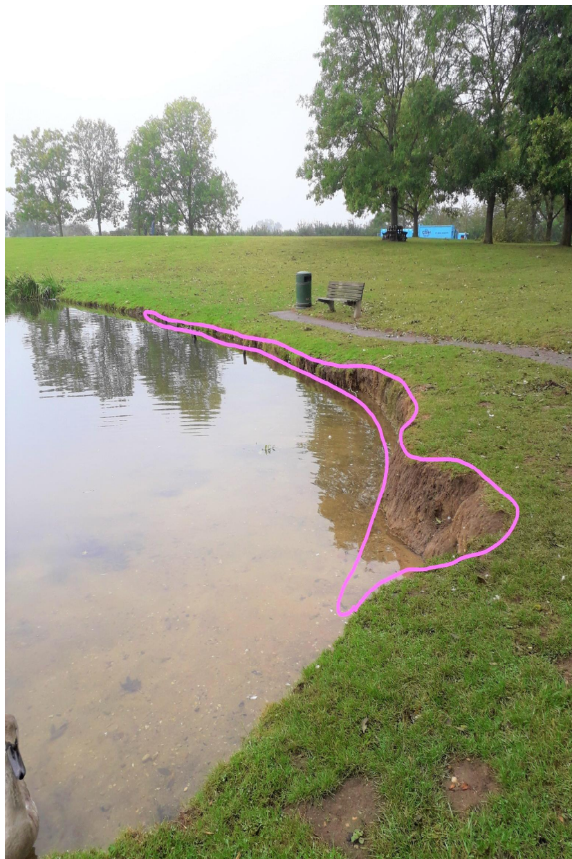
Photo 2 - Stretch of river bank at Caley Green (looking South-West) showing areas of eroded bank (and extent of existing but decaying wooden revetment)
